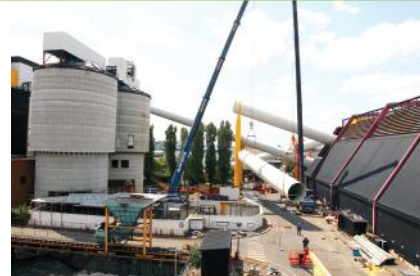
Full scope biomass handling at co-firing plant
