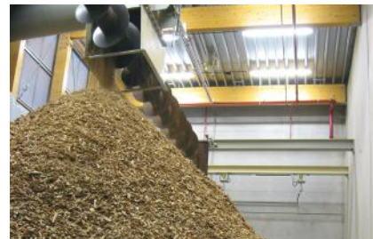
Biomass unloading and storage installation
