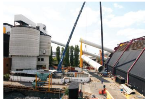
└ Turnkey biomass and coal handling at co-firing plant
