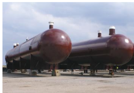
Bullets for the storage of gas
