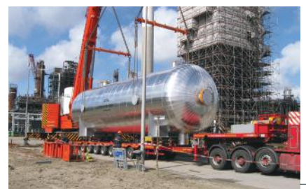
Rapid acid dump vessel
