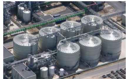
└ Stainless steel tank farm
