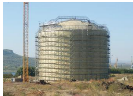
Refrigerated liquid ammonia storage tank
