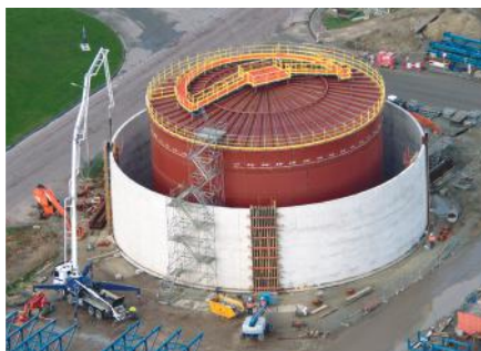
Storage tank with bund wall
