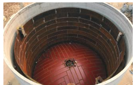
└ Cryogenic double-walled ammonia storage tank
